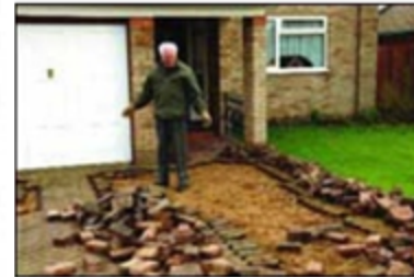
Frank Horsley on his demolished drive
